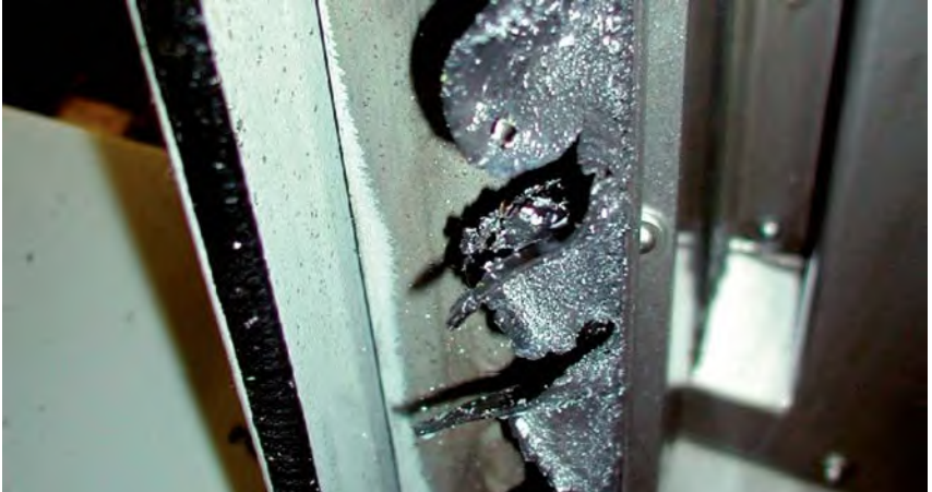
Figure 28 Door sealing not suitable for technical fire prevention and protection
