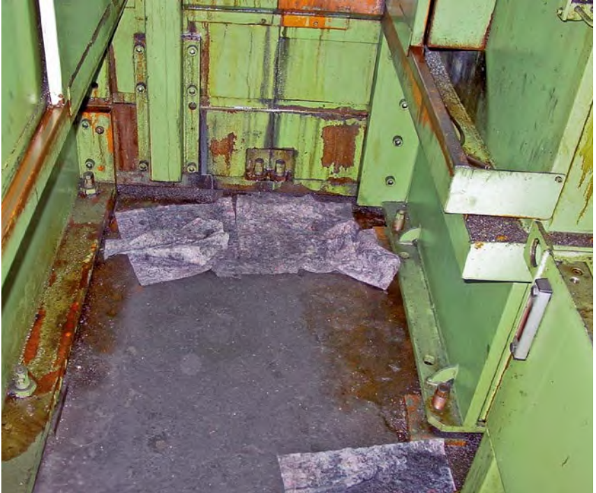
Figure 57 Fire hazard near to a machine
