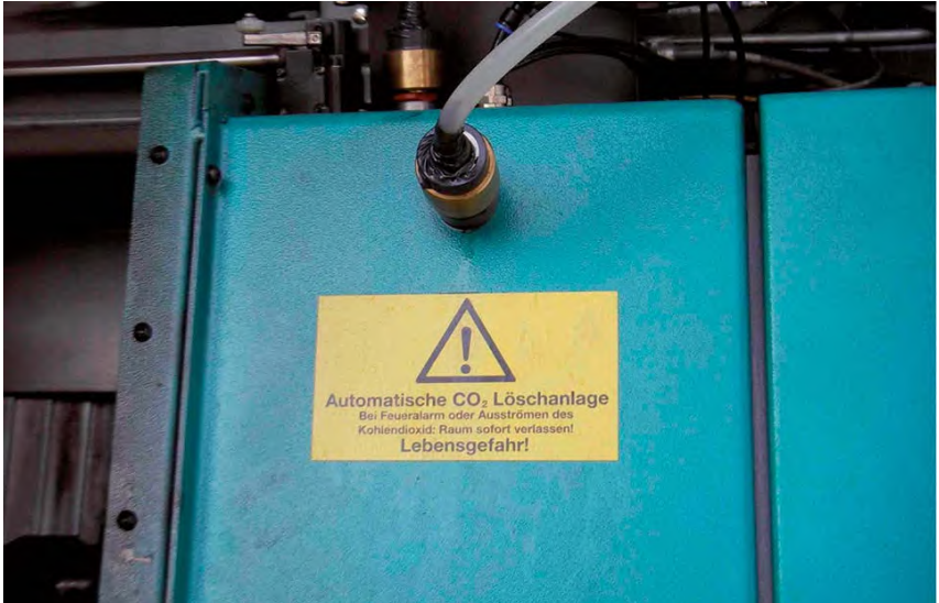
Figure 58 Warning sign for CO 2 extinguishing gas hazards
