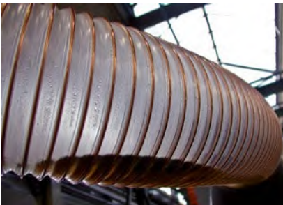
Figure 36 Accumulation of oil in the extraction ducting
