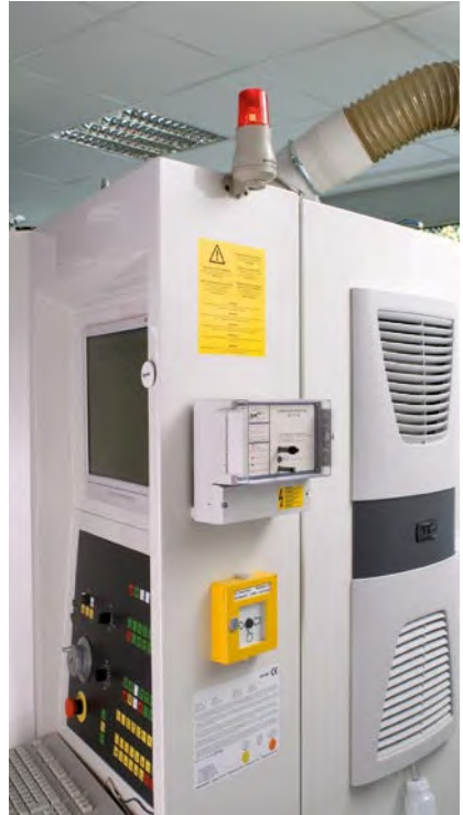
Figure 52 Fire alarm centre with manual activation
