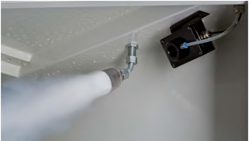
Figure 54 Extinguishing nozzle in operation
