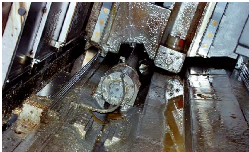
Figure 21 Oil pool formation in the drive room
