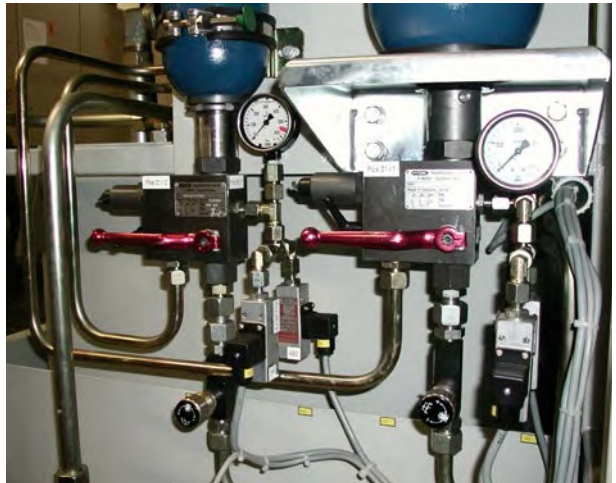
Fig. 25 Depressurized hydraulic accumulators with closed pressure lines
