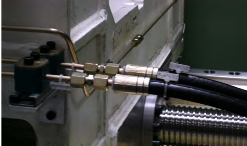
Fig. 26 Markings on pipe and hose side
