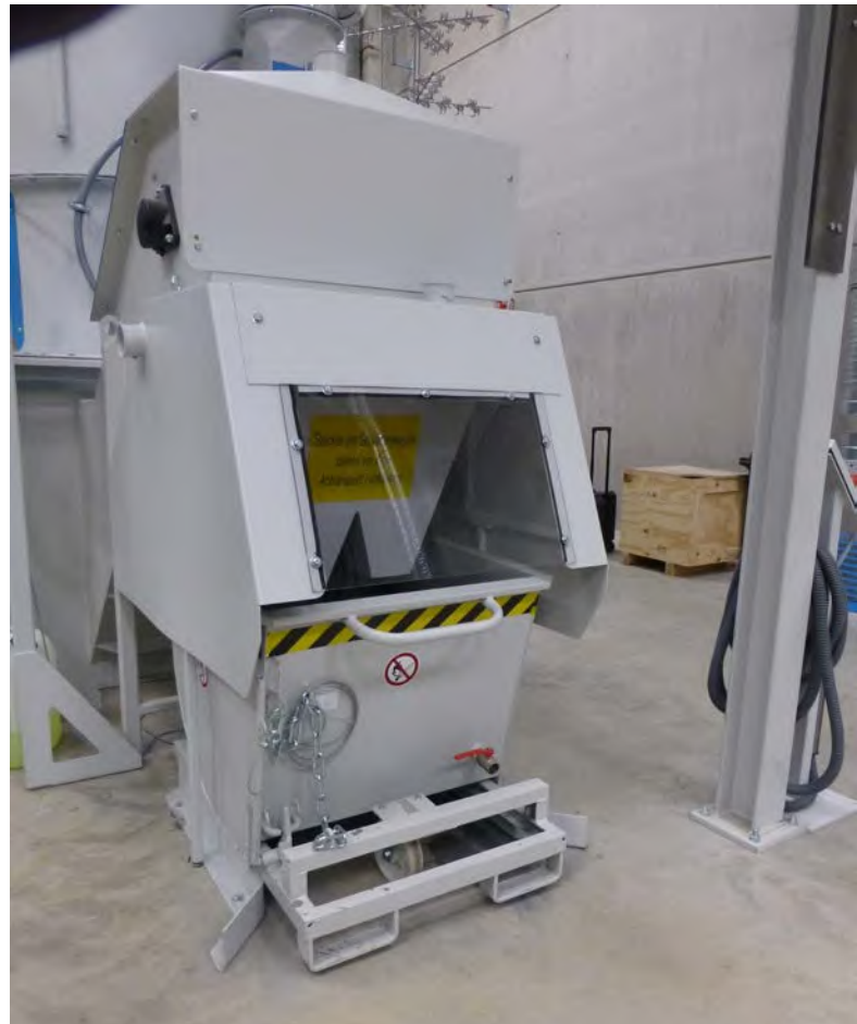
Figure 27 Sludge tipper for magnesium deposits from wet scrubber
