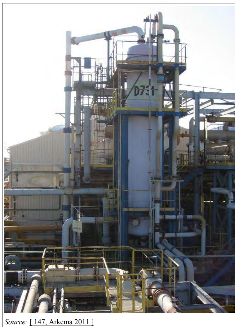
Figure 2.18: View of a chlorine absorption unit
