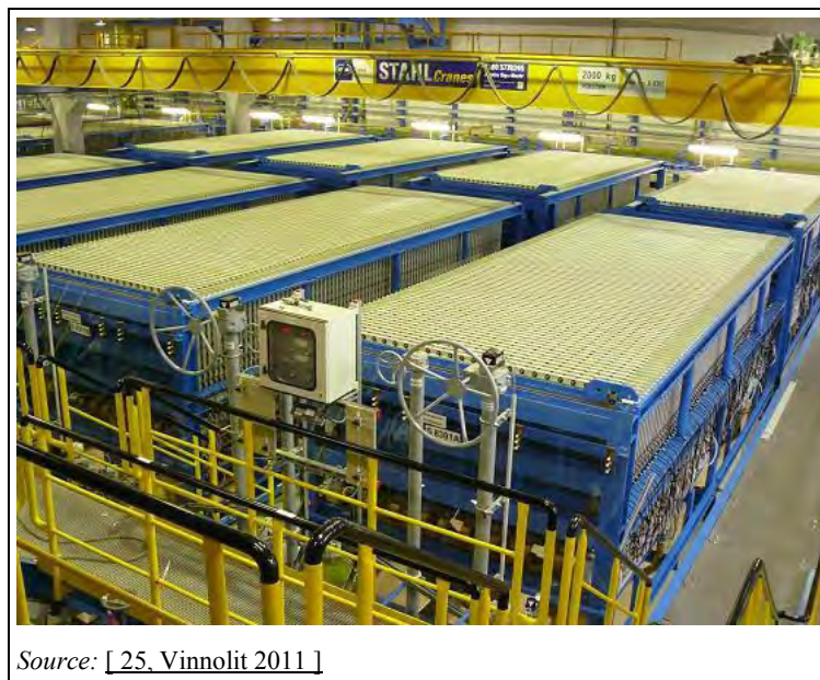
Figure 2.10: View of a membrane cell room equipped with bipolar electrolyzers
