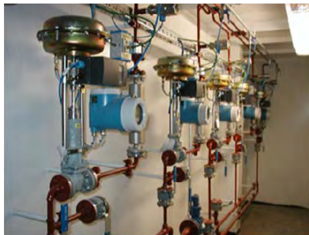
Figure 6.28: Measuring and dosing station with pneumatic valves
