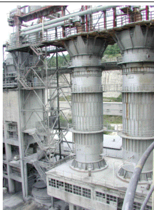
Figure 2.21: Mixed feed shaft kiln
