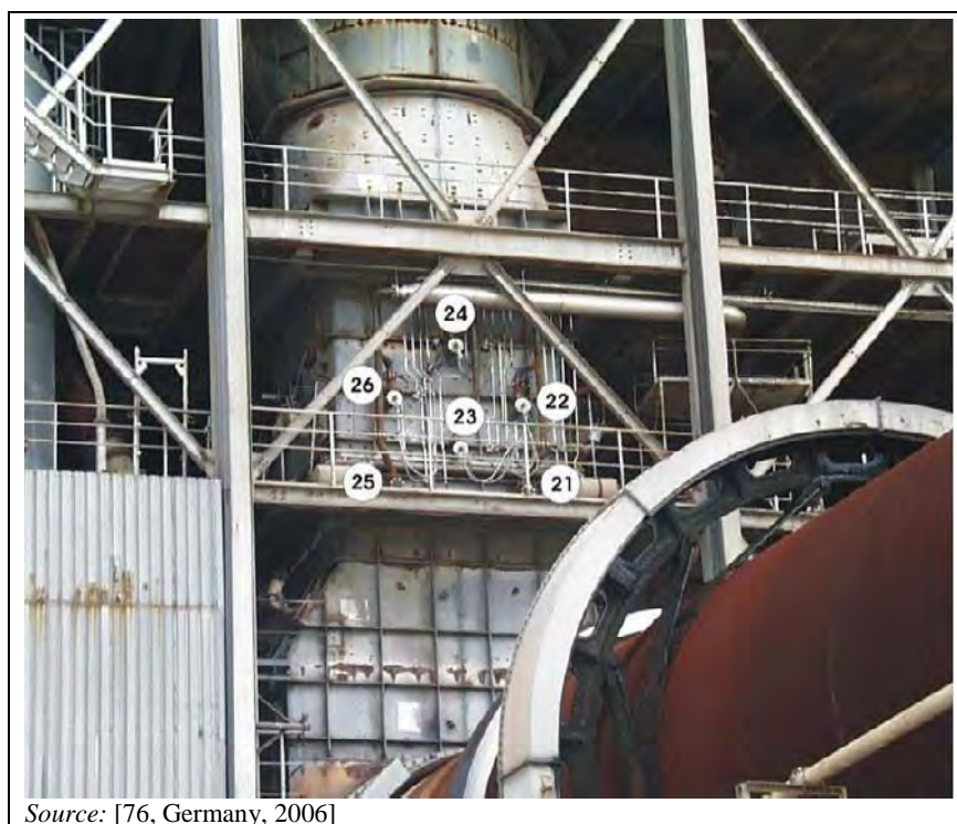
Figure 6.8: High efficiency SNCR and place for injection of ammonia water via lances at places Nr. 21 to 26
