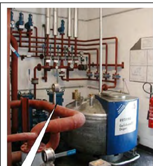
Figure 6.27: Pumping station number 2 with a filter and a waste container for cleaning the filter
