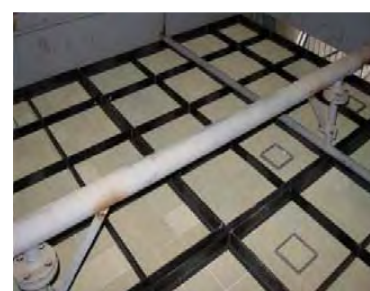
Figure 1.68: Example of a module position used for the SCR technique Source: [140, Italy, 2007]
