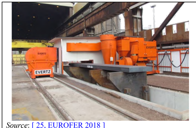
Figure 2.75: Grinding machine equipped with waste gas cleaning abatement system at Tata Steel IJmuiden
