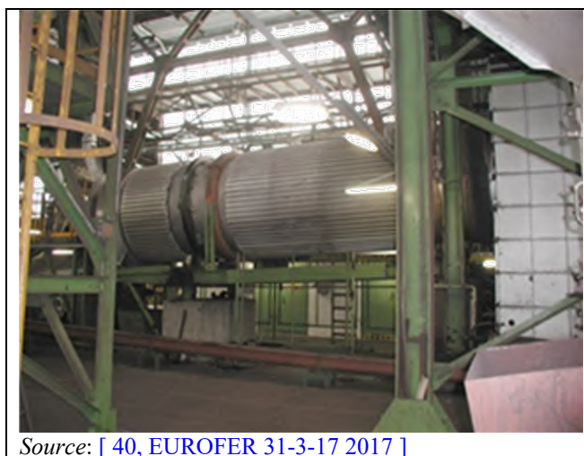
Figure 8.56: Picture of a rotary kiln for thermal treatment of oily mill scale at an ArcelorMittal integrated plant
