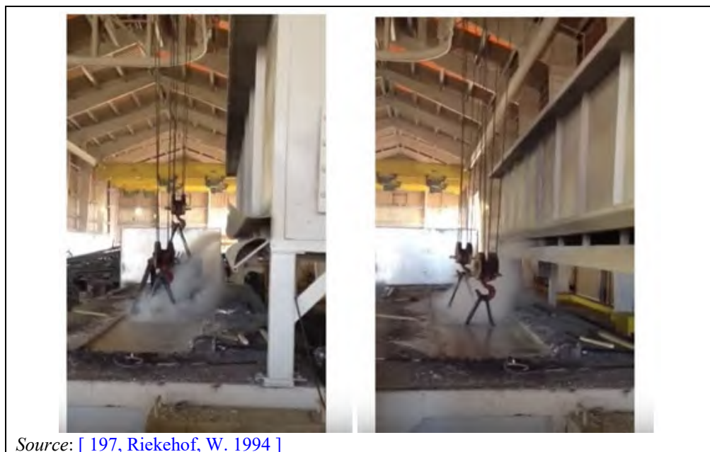
Figure 8.50: Lip extraction at a batch galvanising plant
