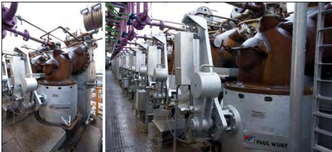
Figure 11.5: SOPRECO Model 2 valves on a stamped charged battery
