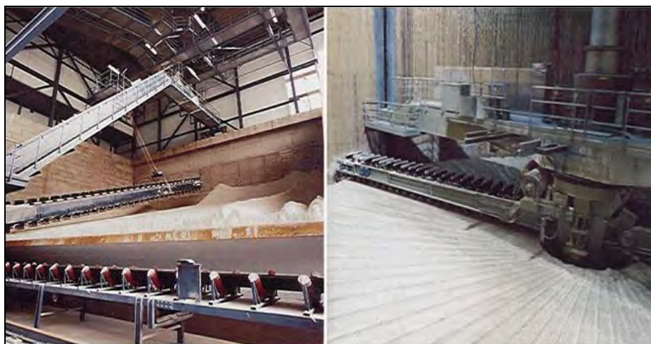
Figure 4.23: Closed gypsum storage facilities [94, Umwelt + Technik, 2000]
