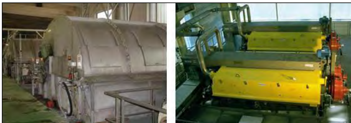
Figure 4.6: Example of a wash filter (left) and a wash press (right) in brown stock washing
