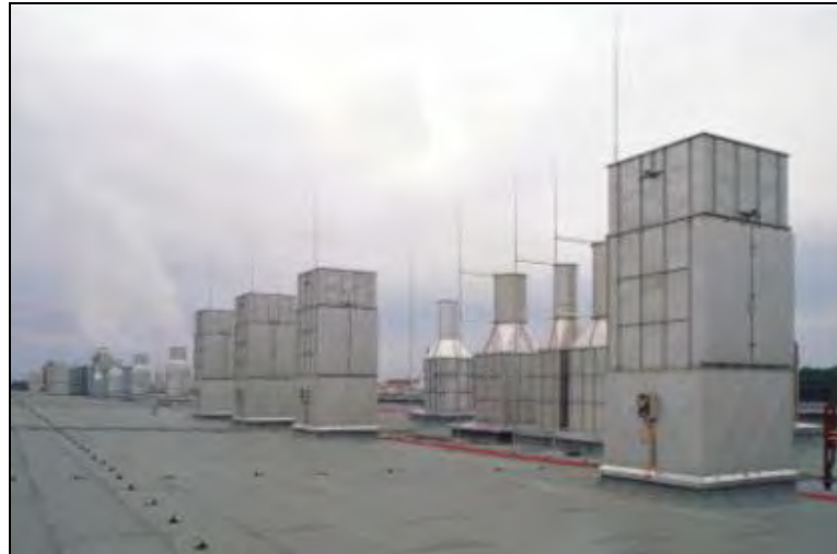
Figure 7.37: Silencers on the paper mill roof
