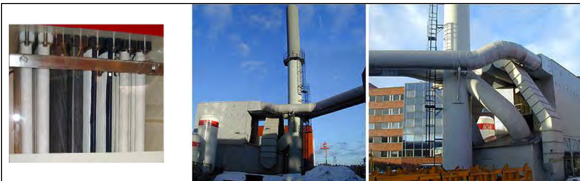
Figure 4.10: Bag filter units; inside (l.) and outside (m., r.) views [237, HUT, 2003]
