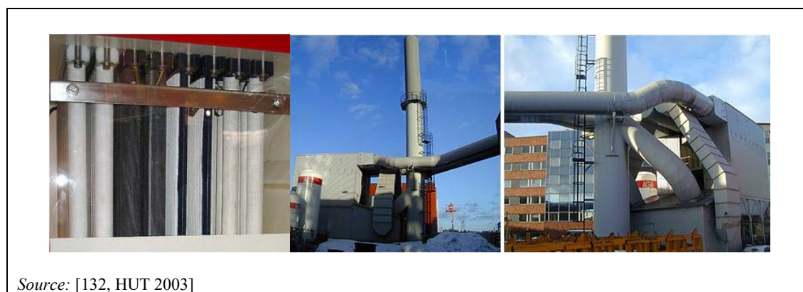
Figure 3.57: Bag filter units; inside (L) and outside (C, R) views
