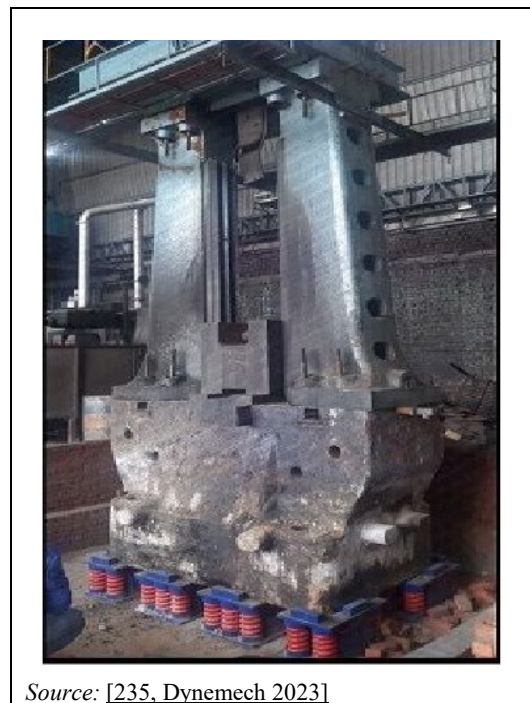
Figure 3.68: Closed-die hammer (3.5 tonne) on spring viscous isolators
