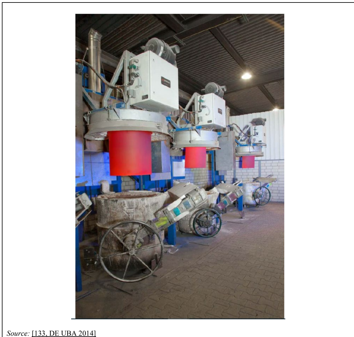
Figure 3.6: Ladle preheating using porous burners
