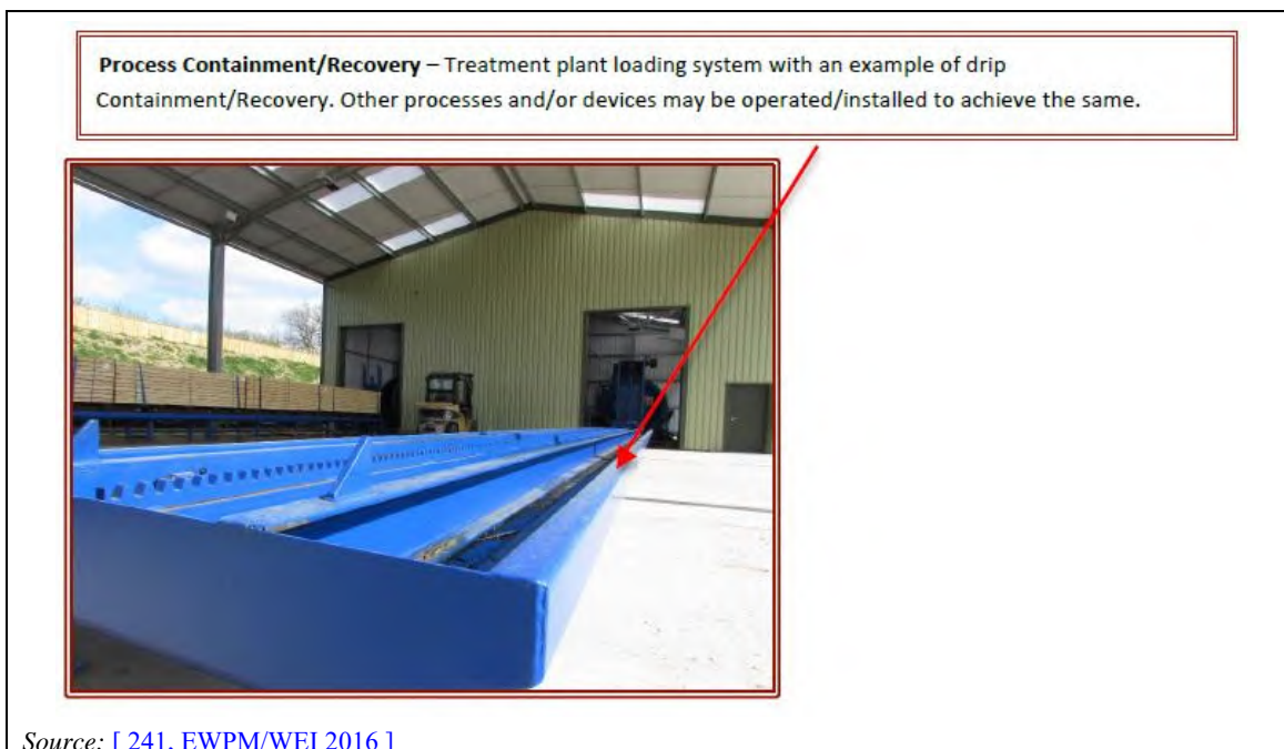
Figure 15.24: Example of a drip tray incorporated into the unloading system (beneath pull-out)
