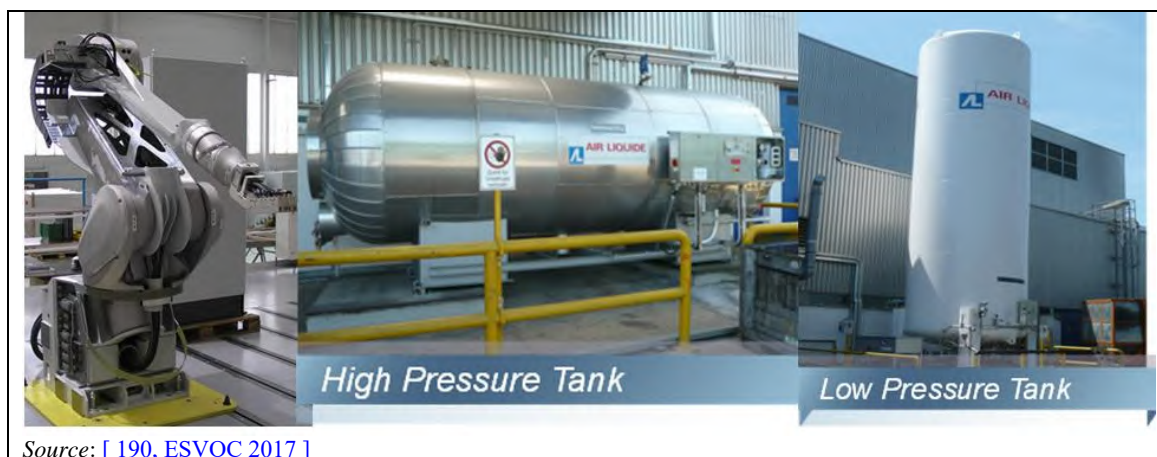
Figure 17.14: (a) Applicator robot, (b) High-pressure CO 2 tank, (c) Low-pressure CO 2 tank
