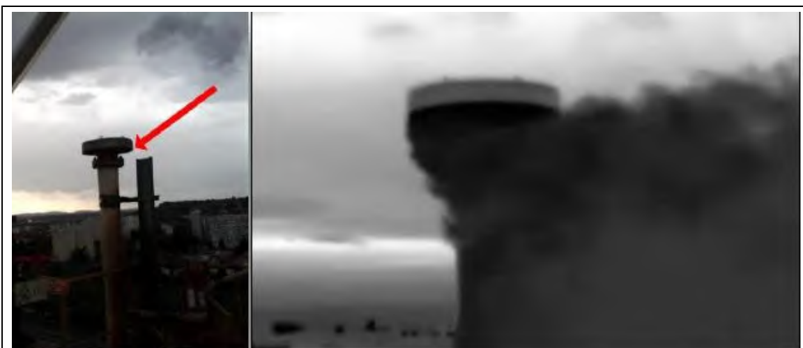
Leak on vent
