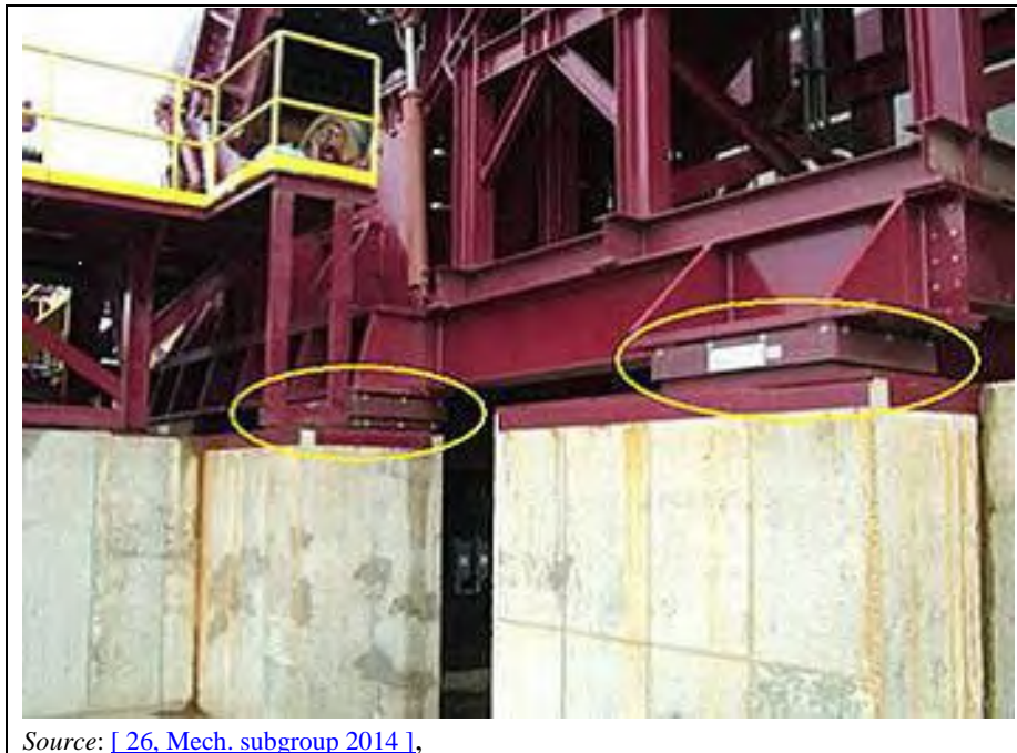
Figure 3.22: Isolation elements (circled) for vibration reduction
