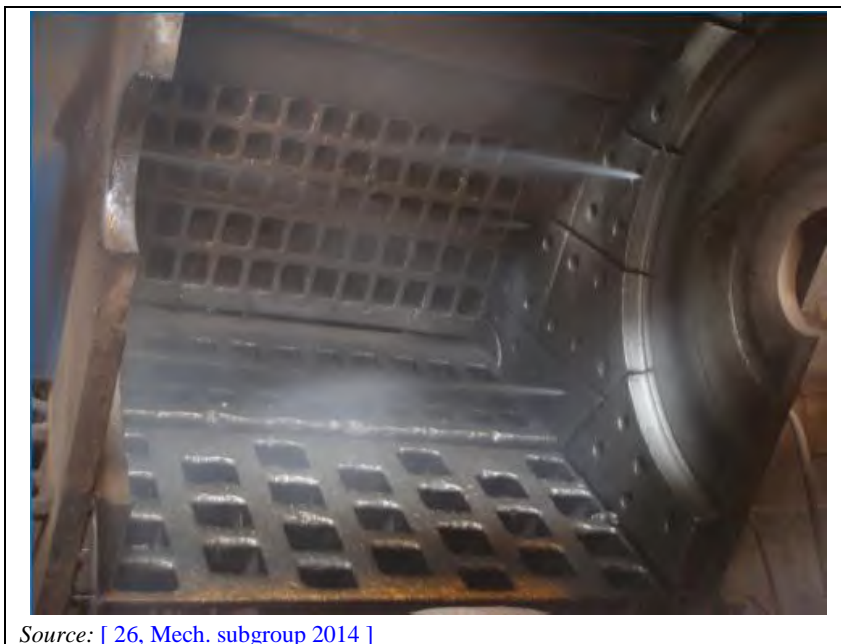
Figure 3.18: Water injection into the shredder mill
