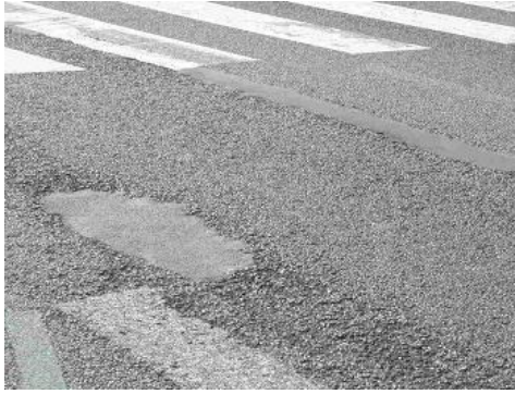
Figure C5 Delamination, fretting and ravelling
