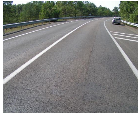
Figure C9 Poor transversal joint
