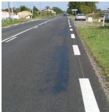
Figure C10 bleeding or fattening up of UTLAC (loss of macro-texture)
