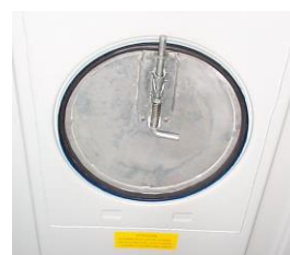
Figure 9.11 Roof hatch internal lock
