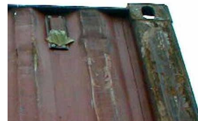
Figure 5.20 Vent tapped over
